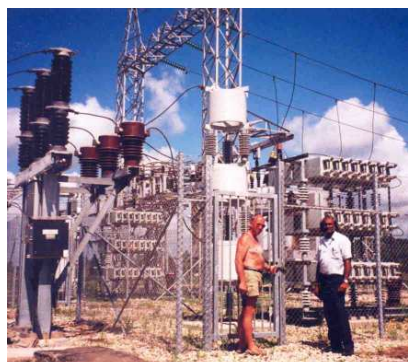
Ubungo Substation 33 kV switch gear
