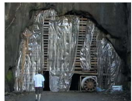
Sandblasting exhaust arrangement
