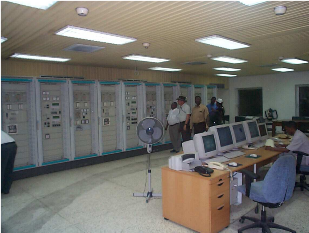
Fig 4.New Computerized Control Room
