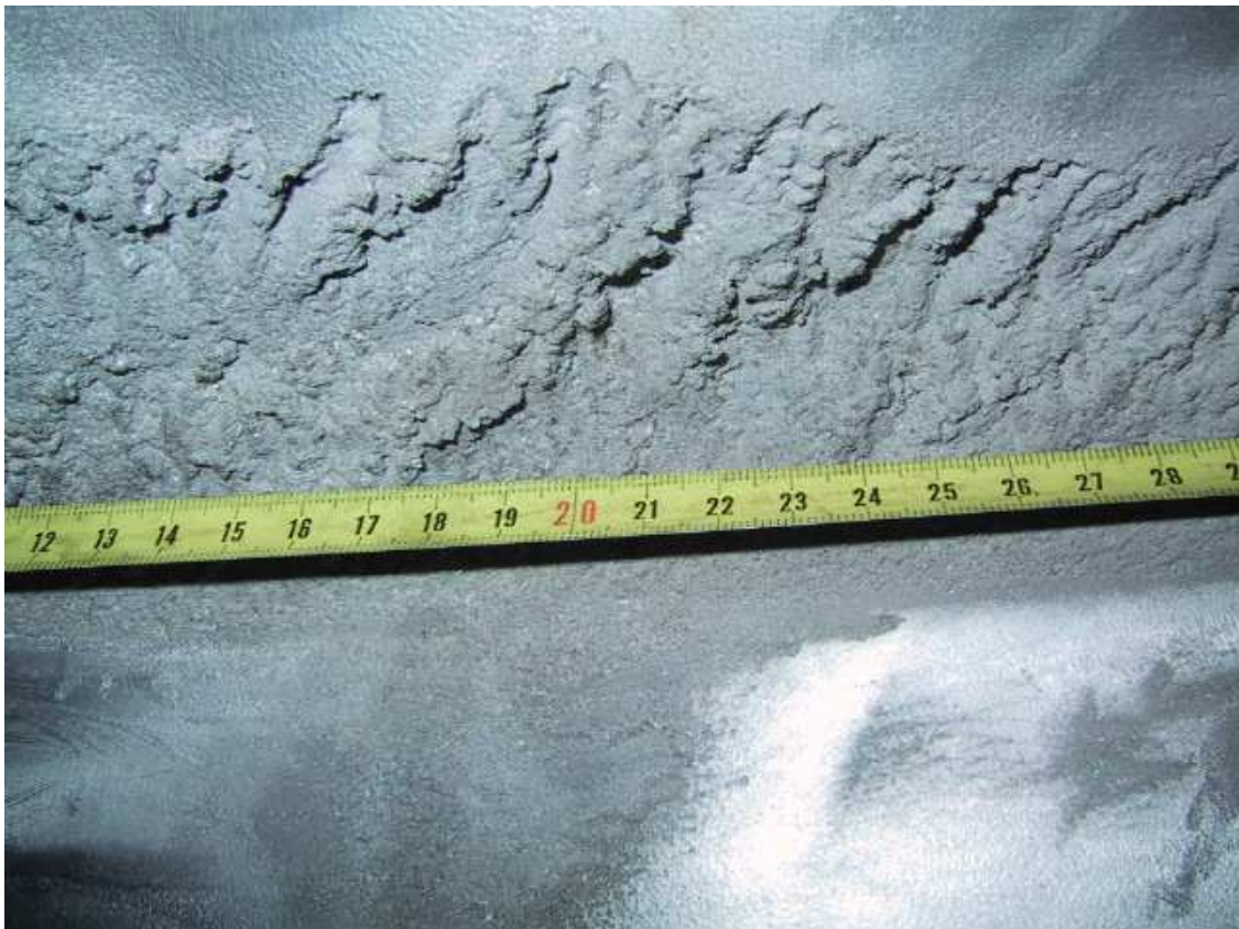
Fig.1 Outlet Cavitations Damage on one of the runner blades
