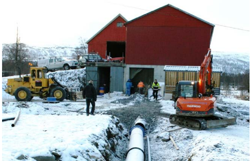
Powerhouse In an old barn
