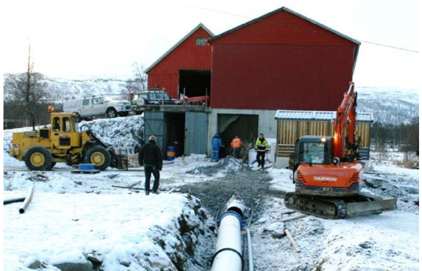
Powerhouse In an old barn
