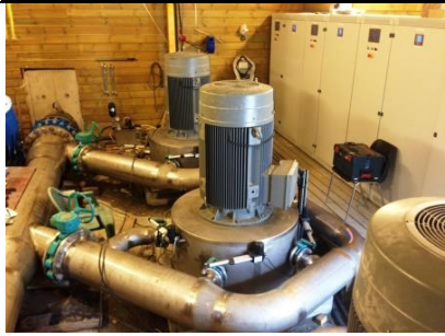
3x160kW Pelton turbiner
